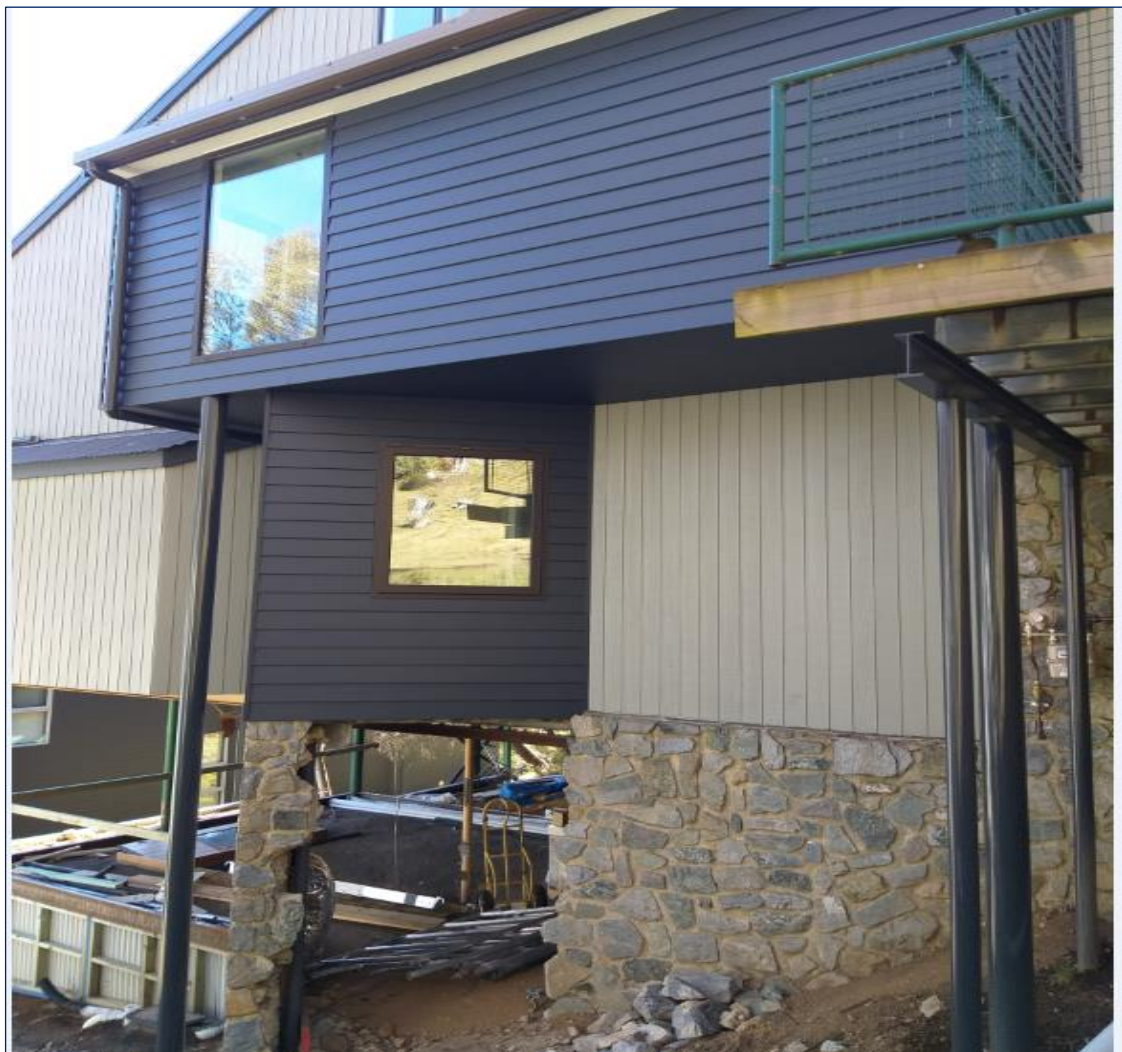
Figure 4 | Construction works September 2020, which illustrates external and basement level works carried out, with basement area uncompleted due to compliance action (Source: Department inspection)
